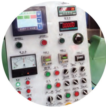
Control Panel with HMI System
